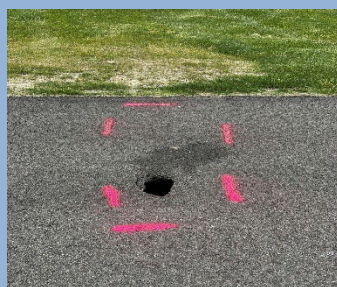
Sink hole on Meadowview Ct.
